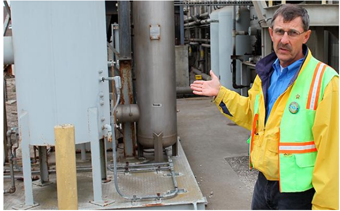
MRWMD General Manager William Merry explains how methane gas released at the landfill is driven into engine generators.
